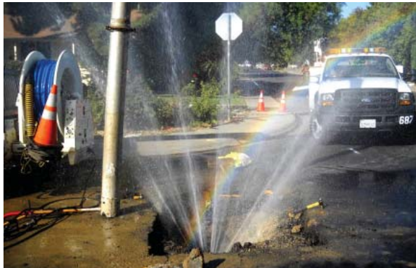
Water main break at Askley Avenue, October 2009
